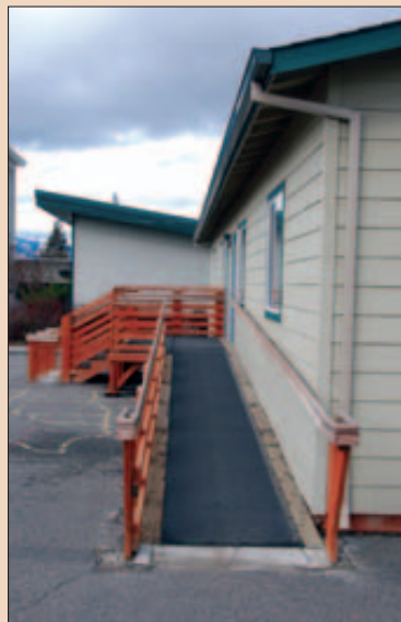
Disabled ramps cannot be installed outside Grade II-listed buildings
